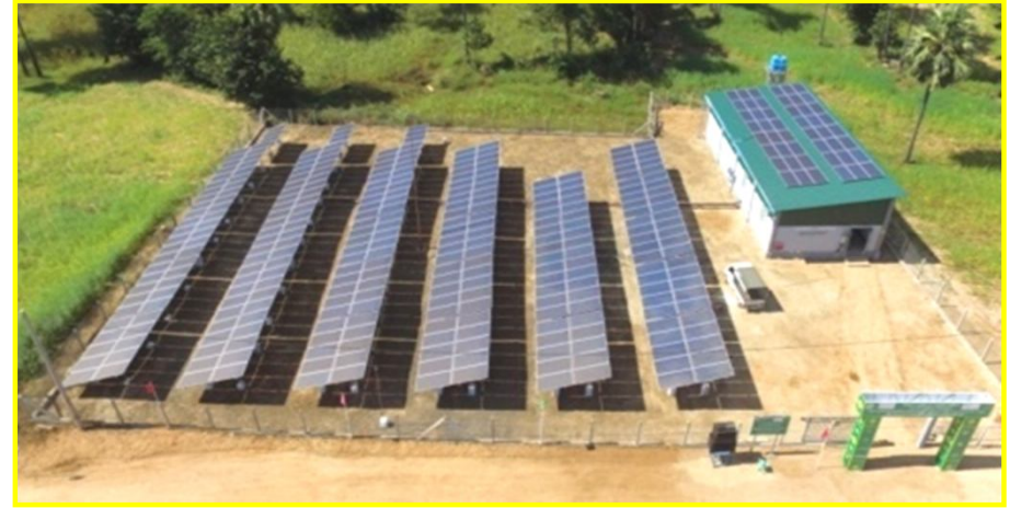
110 kW Solar Mini-Grid System
