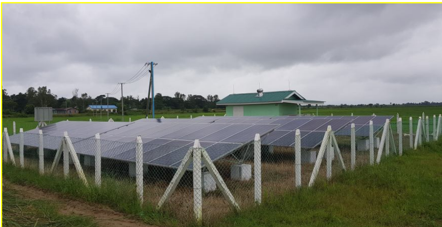
30.72 kW Solar Mini-Grid System combined with 24 kW(Diesel Backup System)
