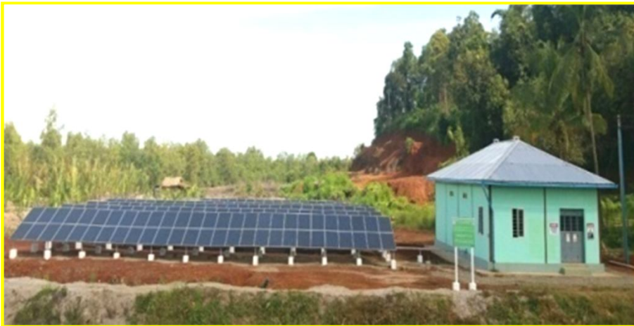
63 kW Solar Mini-Grid System combined with 50 kW(Diesel Backup System)
