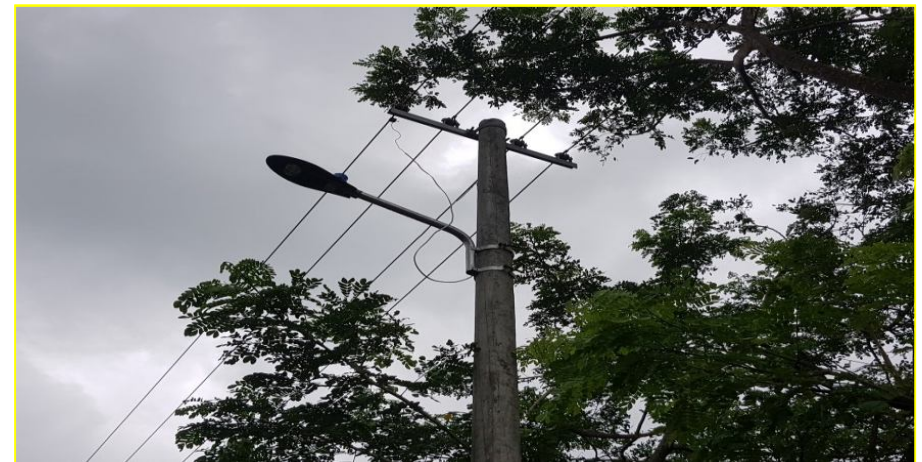
Distribution Line and Streetlight
